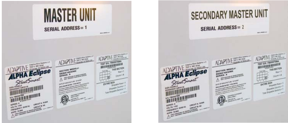
Figure 30. Master/Secondary Master labels
